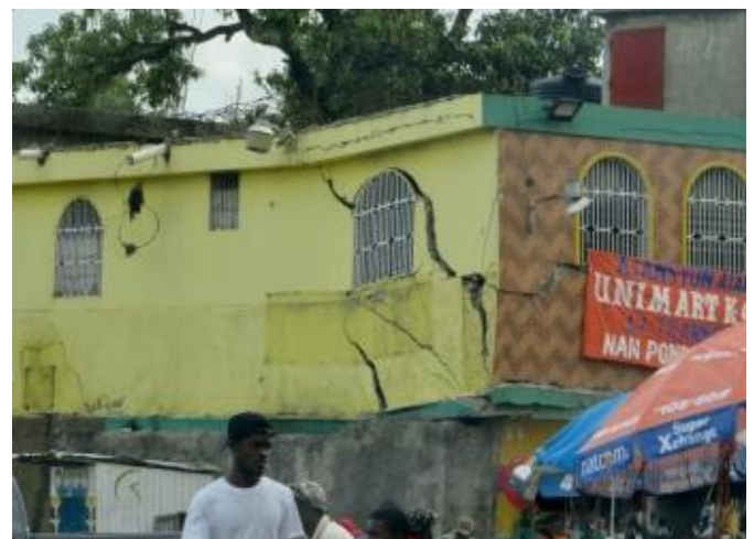
The grocery store we frequented is unstable and could fall at any time.
